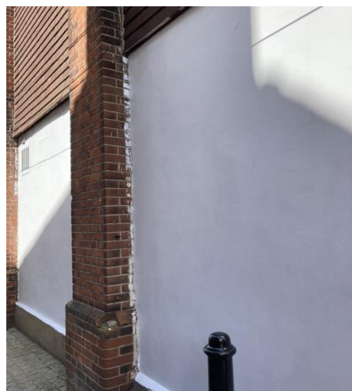
Photo after graffiti removed (June 2024)
